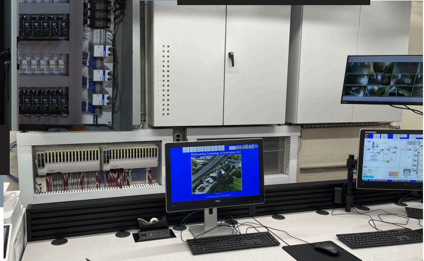
Control Room with Eurotherm T2750
